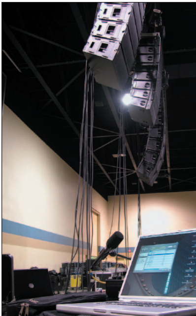
PC at the ready for any processing tweaks.
