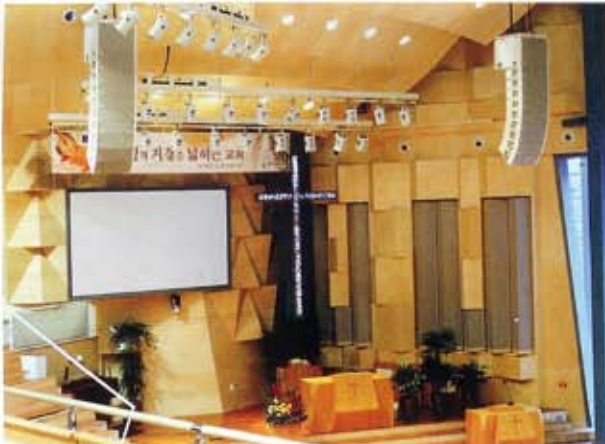
The Adamson SpekTrix FOH sound reinforcement system in position
