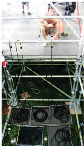
The many on stage performers are fed bespoke cabling via a recess in the stage below
