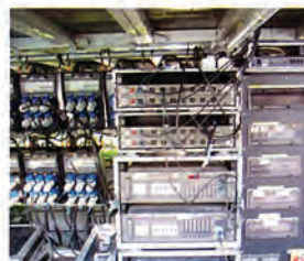
Dimmer and lighting power racks
